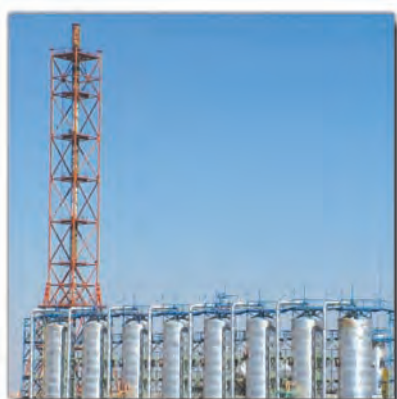
Gas pipelines © Uzexpocenter
